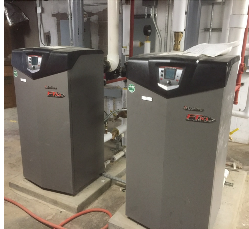
Two 500,000 BTUH Boilers
