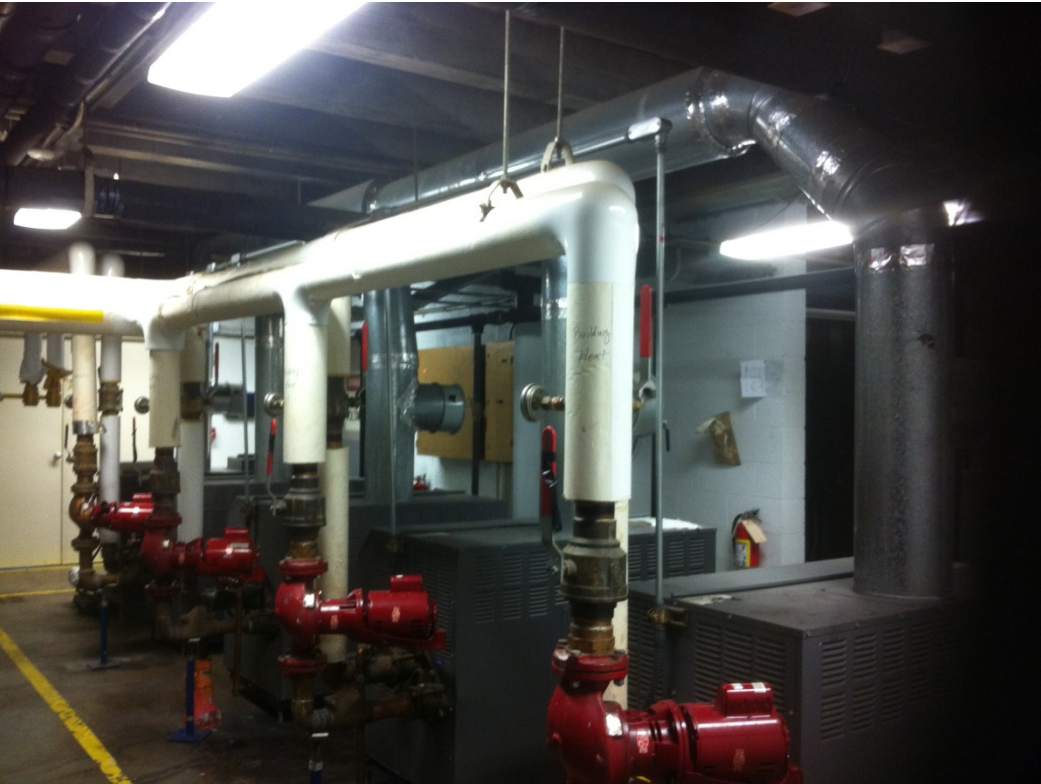
Five 1,000,000 BTUH Boilers
